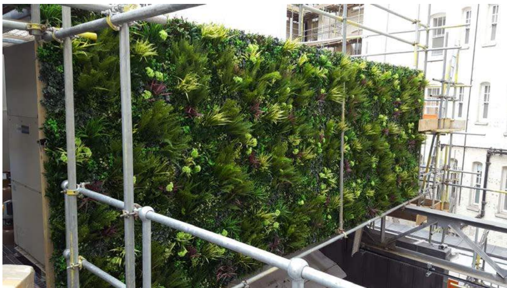
Completed project dressed with Delicate White Colour Box prior to install due to complicated access to the wall
